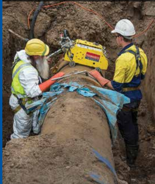
Kennards Hire Pump and Power provides generators to power equipment like Hydraulic Pipe Saws
